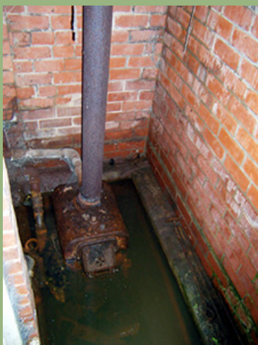
Boiler B2 for Greenhouse G1 See building Restoration
